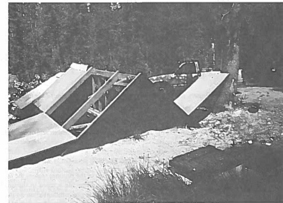
(b) Inlet valve boxes (lower right) and cover over filter with two panels opened.
