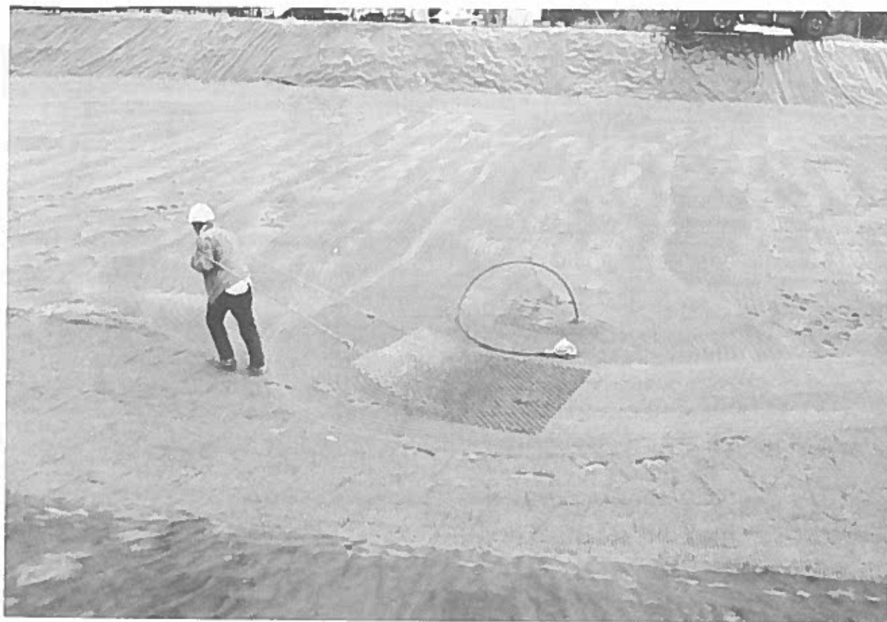
Fig. 4.26 Operator levels the sand surface with a section of chain-link fencing (Source: Cashmere, WA Slow Sand Filter, photo by Steve Deems, Washington Department of Health)
